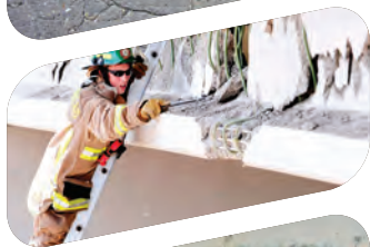
Mechanical - Impact Damage
