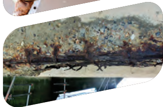
Chemical - Steel Corrosion
